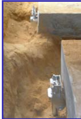
Before and After Views of Replacing Failed Auger Cast Piles with Drive Rite™ Helical Piles for Parking Deck
