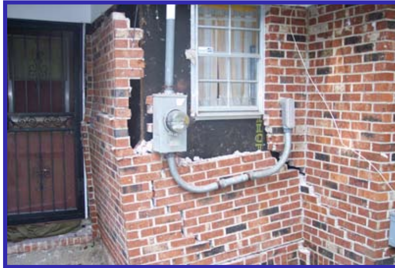
This Section of the Residential Home Collapsed into a Sinkhole
